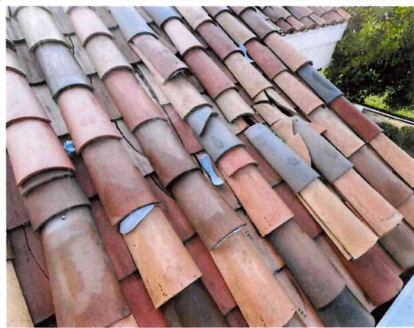
Tile damage: Broken tiles and localized exposed roof areas.
