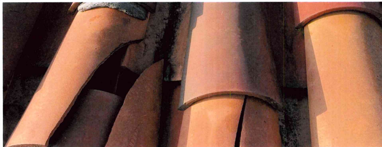
Close-up: Cracked and broken mission-style roof tiles.
