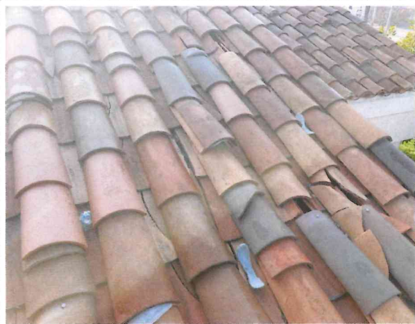
Tile damage: Displaced and fractured tiles with visible prior repairs.
