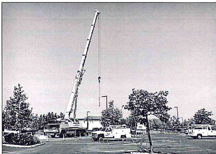
Crews from the Metropolitan Water District of Southern California and the Eastern, Western and Temescal Valley water districts use a large crane as they repair a state-operated pipeline that was leaking in Moreno Valley on Friday.
